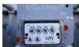
Automated Meter Reading
